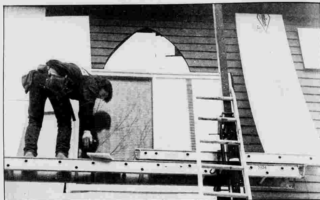
HOME IMPROVEMENT — Brian Mawdsley of Hebron installs vinyl siding Tuesday at the Samaritan Shelter at 466 Main St. Mawdsley works for Bushnell Home Improvement in Bolton.
