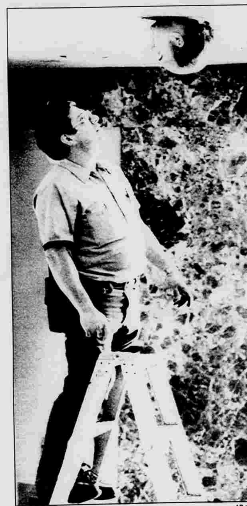
HEADS UP — Ken Brokaw pokes his head through the ceiling to talk to Ray Corey as the two install a light fixture in the lobby of the Lincoln Building in downtown Spokane, Wash., on Thursday.
